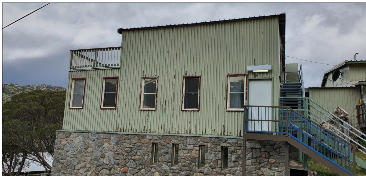
FIGURE 1 EXISTING DETERIORATED CLADDING TO BE REPLACED
